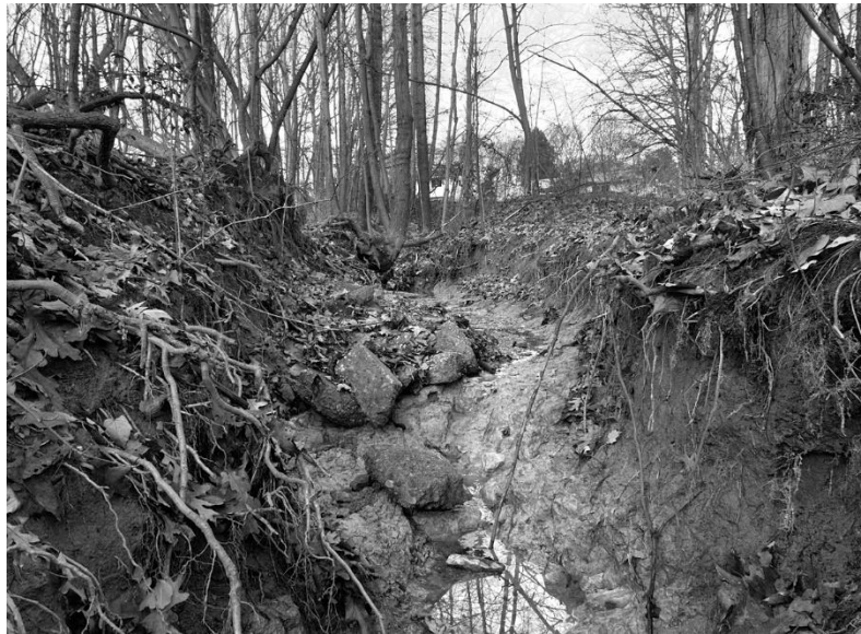
Figure 1. Erosion caused by a storm drain, Royal Lake Park, Fairfax, VA.
