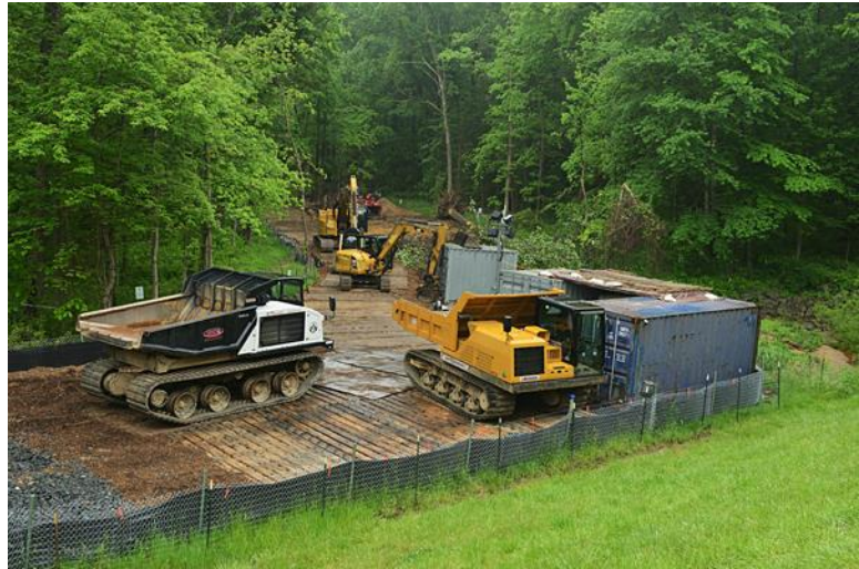
Figure 1. The construction entrance at Roberts Road has a staging area (foreground). Wood planks protect the soil from earthmovers traveling along the work zone.
