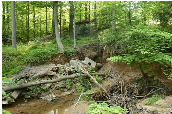
Figure 1. This “before” image reveals the destroyed storm drain outfall and massive erosion next to private property.
