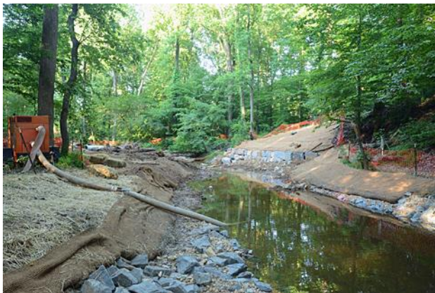
Figure 6. To temporarily reduce the creek's water level for work on that stretch, a pump (left) bypassed water to a down-stream location. Daces and other minnows soon returned.
