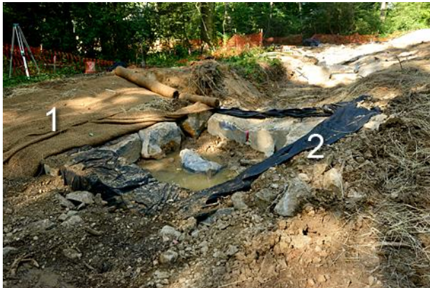
Figure 4. Restoration typically goes in a downstream direction. This incomplete section shows the coir nets (1) unrolled to retain soil. Whereas the county is moving away from plastic materials in restoration projects, synthetic geofabric (2) lines the waterway bottom with boulders and pebbles on top.
