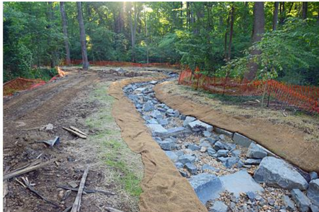
Figure 5. Near the outfall, the waterway is finished. Boulders and a curved course reduce the rushing storm water's energy. The interim roadway (left) remained in use until completion of all major earthmoving activities.
