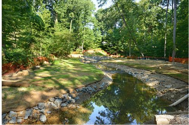
Figure 9. The preliminary work for this stream restoration is done. A shallow streambed allows water to dissipate energy across a wide surface. Grass is already sprouting along the banks. The orange work zone fence will soon come down. After adding native plants in the cool-season months, the reforestation begins—a process that continues for many decades.
